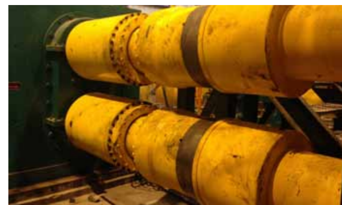
Gear spindles on site
