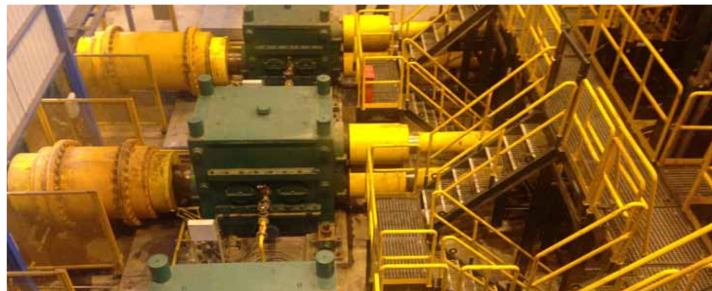
Roughing mill drivetrain
